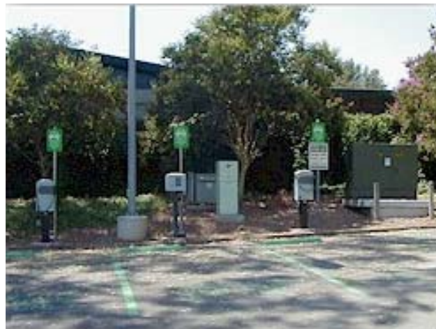
Figure 5-17. Electric vehicle charging station fed directly from utility transformer.
