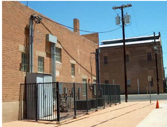
Figure 5-16. Typical commercial electrical supply panel.
